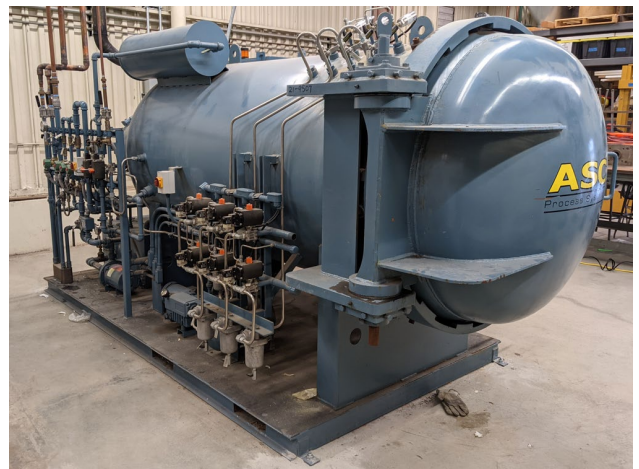
Fig. 11-0-2: Autoclave Front - RHS
