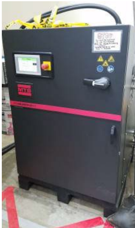
Fig. 5-0-2: MTS Hydraulic Pump
